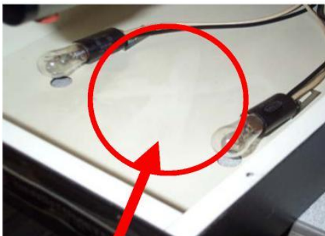
Dirty reflector area
